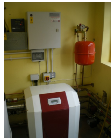
14kW ground source heat pump which provides all space heating and domestic hot
